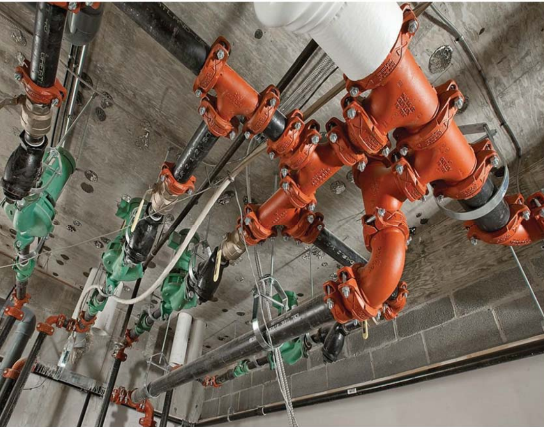
In-line pumps are used for the boiler circulating pumps in a primary/secondary hot water heating system installation.
