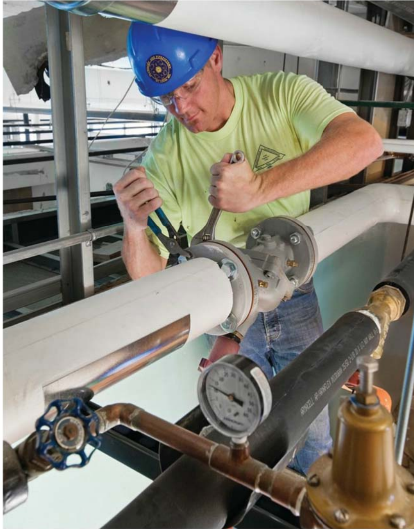
Top: Jarrell pipefitter Tom Reiter completes the installation of a circuit setter. Balancing valves were installed at the top of each of the chilled water and heating hot water supply risers to assist in the balancing of the systems. Bottom: The complete chilled water system at Council Tower, including Taco KV Series pumps with suction diffusers, multi-purpose valves, a bladder-type expansion tank and an air/dirt separator.
