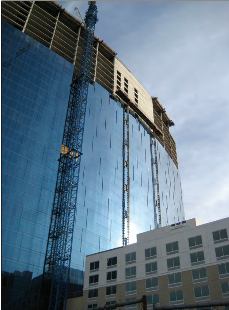
North Mechanical Contracting chose Anvil's Gruvlok product to stay on time and within budget for a new luxury JW Marriott hotel and convention center in Indianapolis (shown here under construction)—which is now ready to welcome more than 100,000 people when Super Bowl 2012 kicks off.
