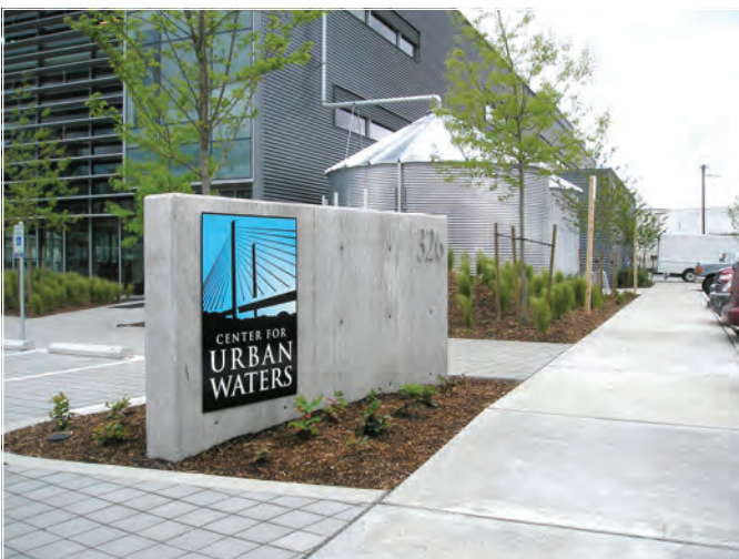
Eagle Harbor Mechanical installed a rainwater harvesting system in Tacoma, WA's Center for Urban Waters building, relying on Jay R. Smith Mfg. Co. products to do the job. The visible stainless steel water storage tanks draw attention to rainwater harvesting and the city's efforts to promote sustainability.
