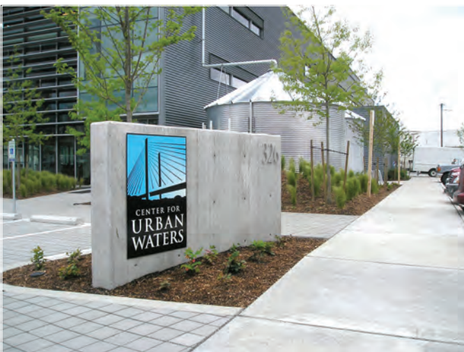
Eagle Harbor Mechanical installed a rainwater harvesting system in Tacoma, WA's Center for Urban Waters building, relying on Jay R. Smith Mfg. Co. products to do the job. The visible stainless steel water storage tanks draw attention to rainwater harvesting and the city's efforts to promote sustainability.
