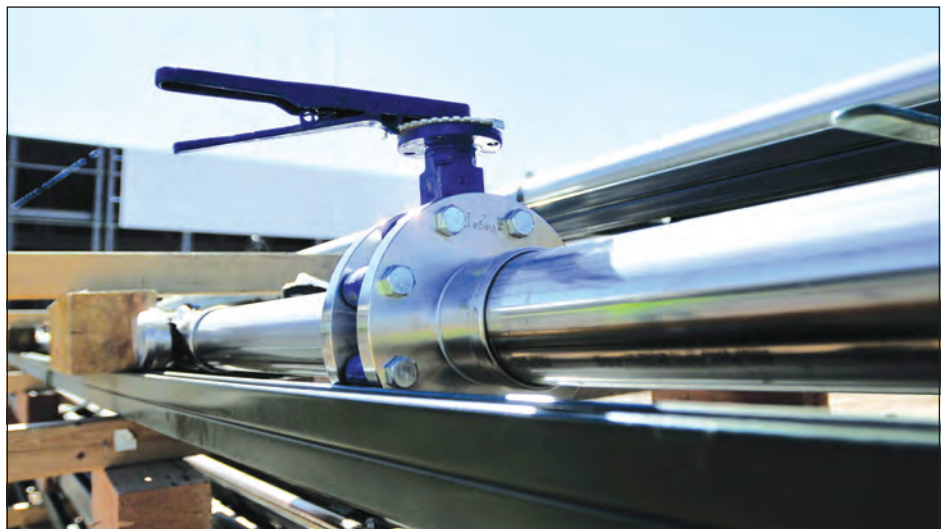
Olson Heating and Plumbing knew Viega ProPress Stainless fittings—with their patented Smart Connect® feature that makes it easy to spot unpressed connections—would be ideal for the new Vestas wind tower manufacturing plant.
