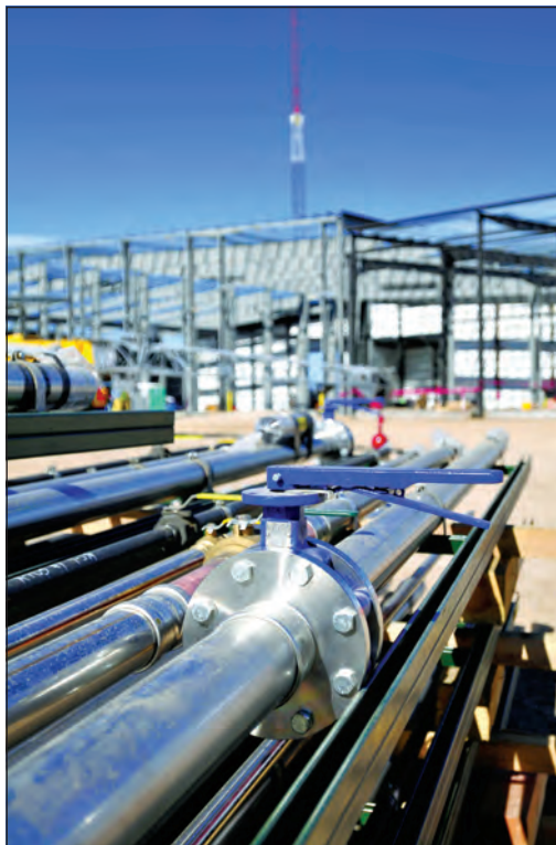
When Vestas Wind Systems began building the world's largest wind tower manufacturing plant, Olson Plumbing and Heating used Viega's ProPress Stainless fittings to ensure that installation of the industrial gas and compressed air portions of the massive project was completed in just five months.
