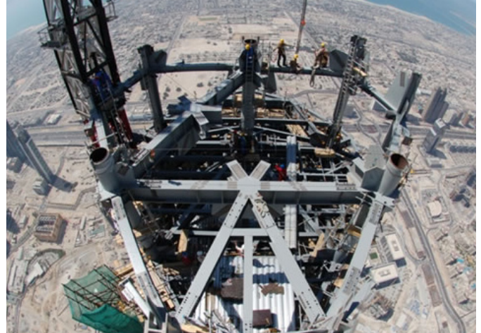
A bird's-eye view of the tower construction on the Burj Khalifa, the tallest building in the world.
