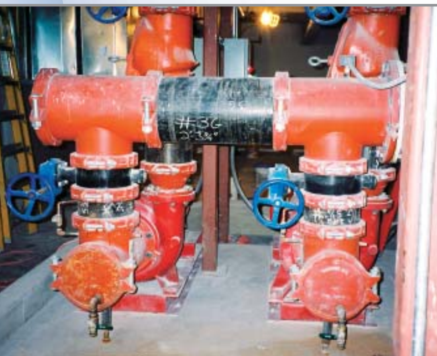
Utilizing limited space efficiently.
