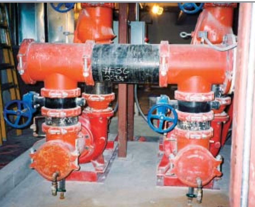
Utilizing limited space efficiently.
