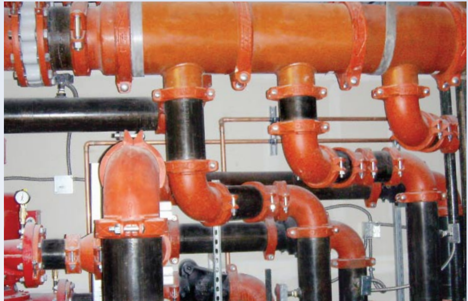
Right: The combination of geothermal energy and Gruvlok® products has reduced the Speedway's electrical usage by 60 percent and maintains an air conditioning capacity far larger than the 90 tons required by the media center.
